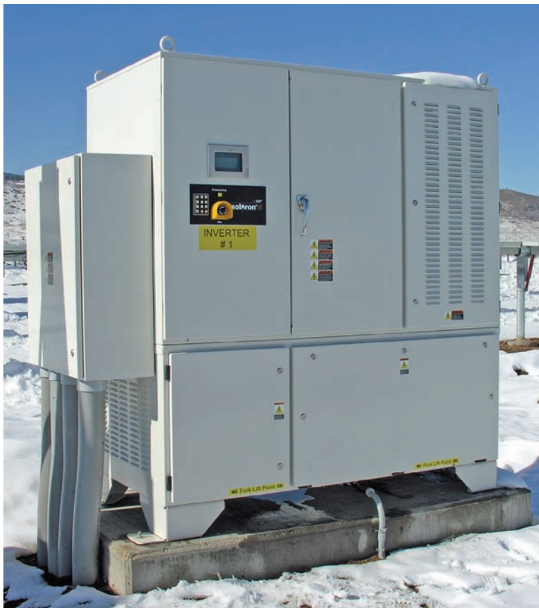
Courtesy, Advanced Energy
