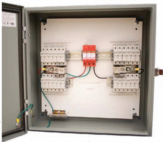
Combiner with surge arrester This SolarBOS 1,000 Vdc combiner is configured for a floating array. Grounded array configurations are also available. The three modules of the DEHNguard SPD are arranged in a fault-resistant Y circuit.
