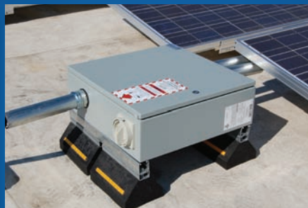
Disconnecting Combiner Boxes
