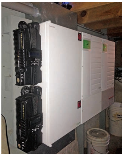
A MidNite Solar Classic 200 MPPT charge controller for each PV subarray. One controls a relay for the water heater diversion-load circuit.
