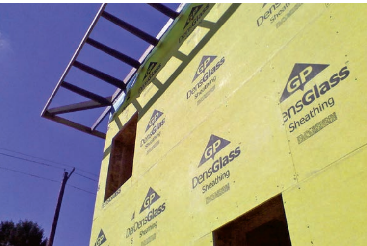
Exterior sheathing is DensGlass fiberglass-faced gypsum for moisture protection—it rains quite a bit in Portland, Oregon.
